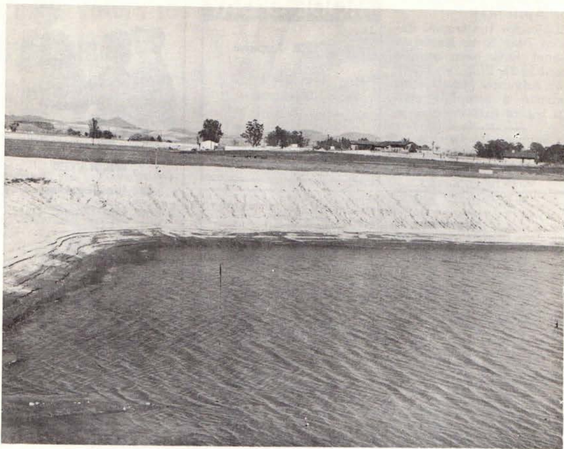
One end of the newly constructed 600-foot reservoir with a capacity of 14 acre feet of water. See the main house in the distance with the guest house at the right.
