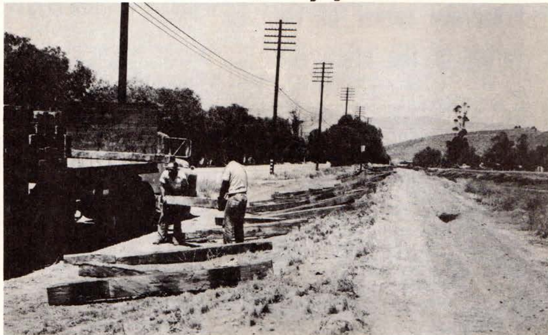
The final scene . . . the ties of the Santa Fe Railroad Avenue line being hauled away
